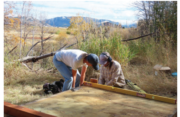
Cathy Stamm & Kevin Cox preparing base for storage shed Photo: Terri Narotzky
